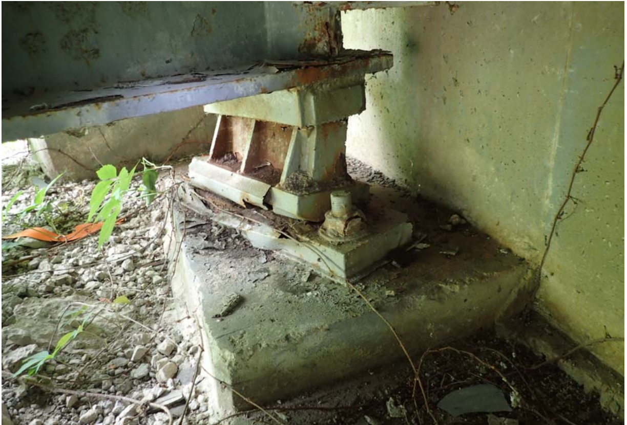
Downstream bearing at abutment 4; Flaking paint with some minor to moderate corrosion.
