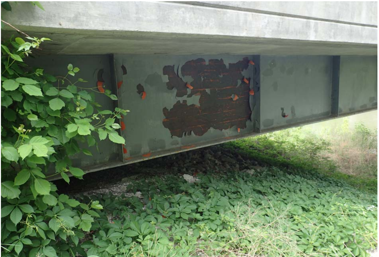
Large area of paint failure on the exterior face of the downstream girder near abutment 4.
