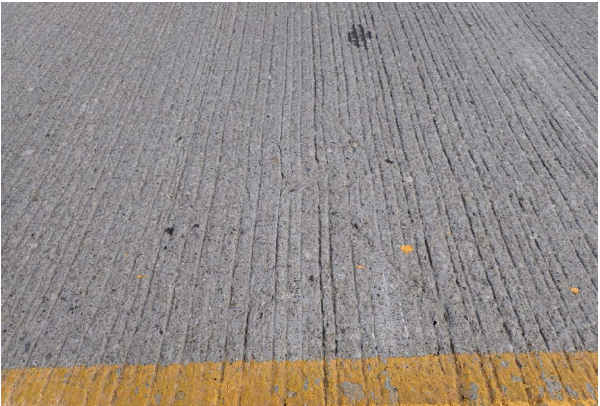
View of minor sized transverse cracking in the wearing surface near pier 2.
