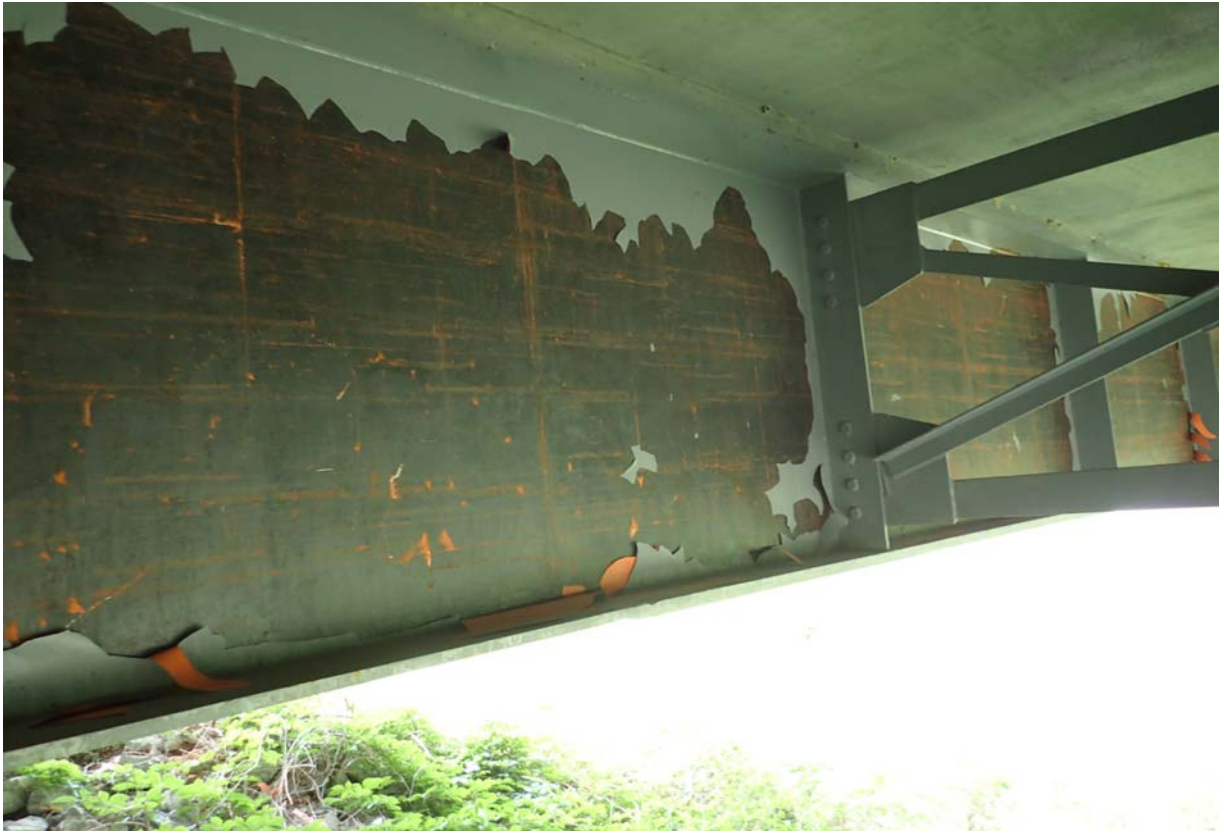
Large area of paint failure on the downstream face of girder 3 from upstream near abutment 4.
