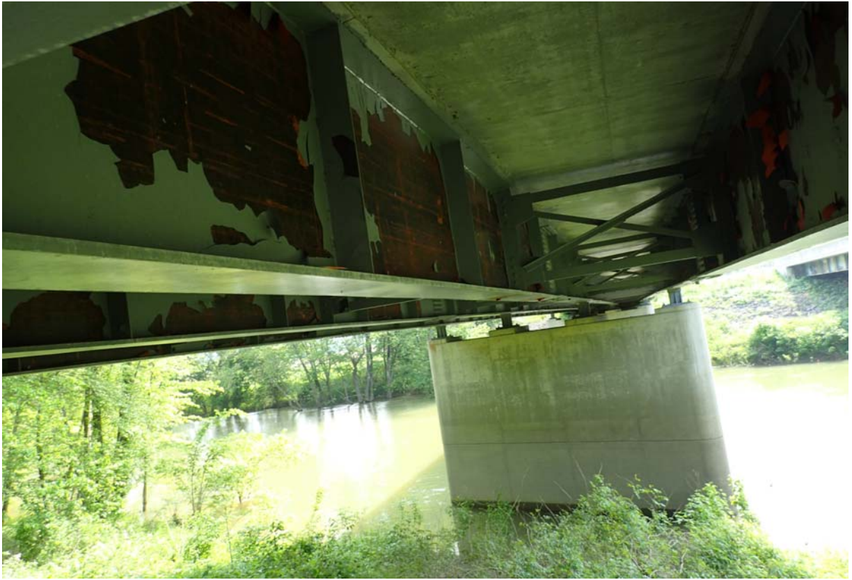
View of several large areas of paint failure on the upstream face of girder 2 from upstream in span 1.
