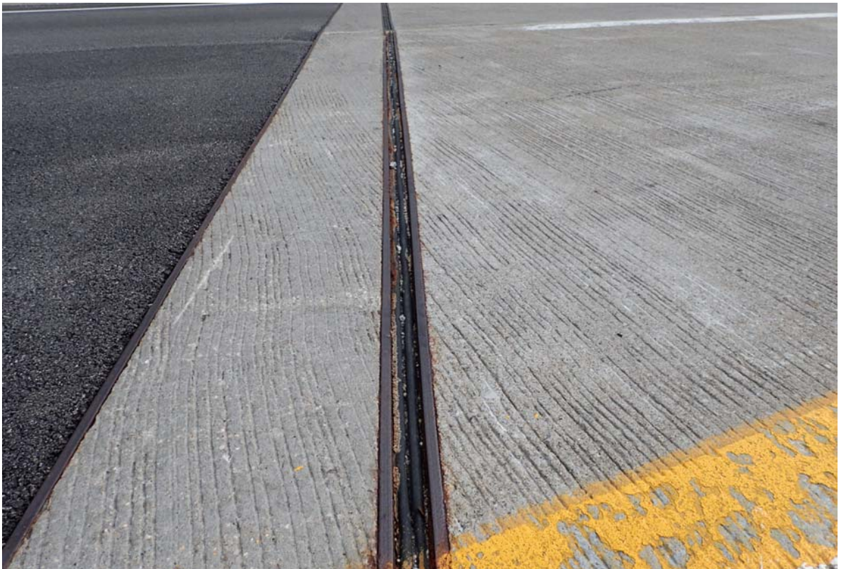
Typical view of the transverse joint at abutment 1; it is partially full of debris, and has some adhesion failures.
