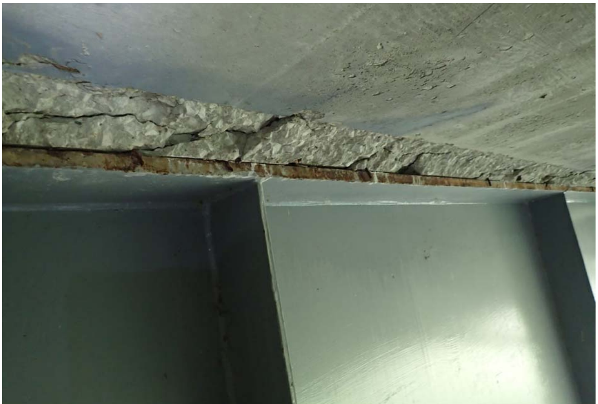
Moderate spalling along the fillet on the top interior flange on the upstream girder at abutment 4.
