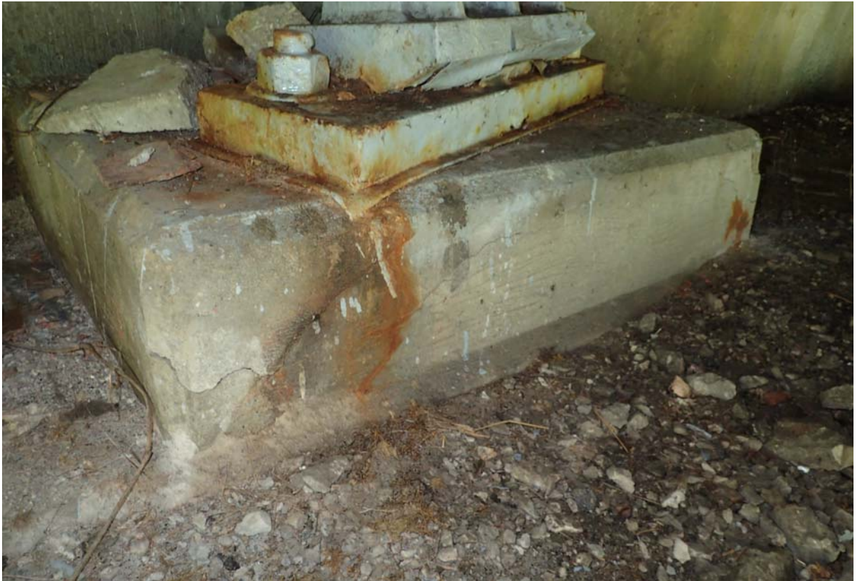
View of some minor cracking of pedestal 2 from upstream at abutment 1.
