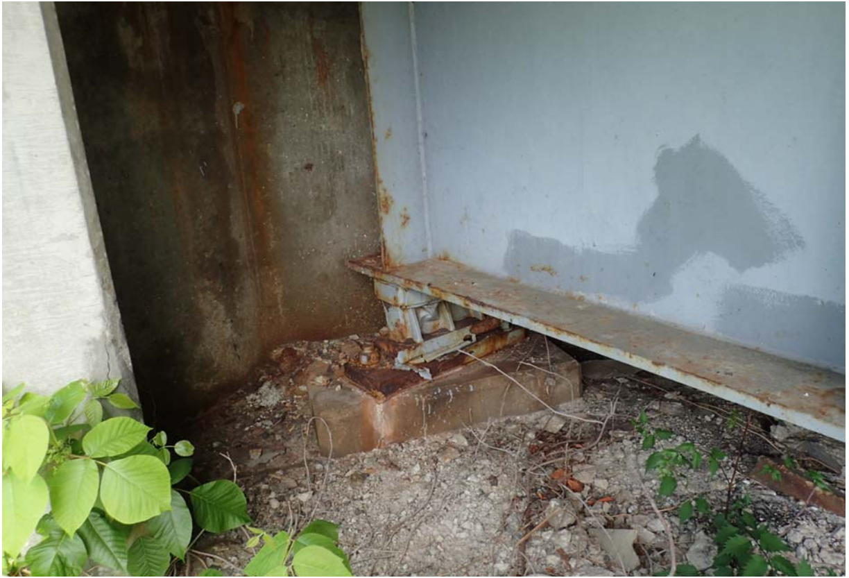
Upstream bearing at abutment 1; flaking paint and moderate corrosion.
