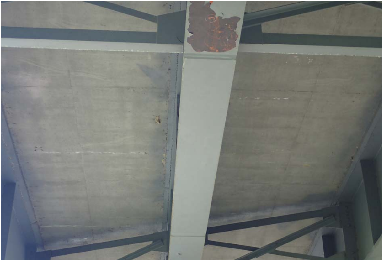
View of minor cracking with efflorescence in the deck underside at pier 3.
