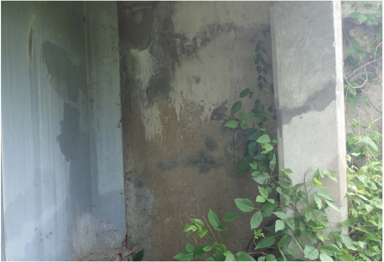
View of minor cracking with efflorescence in the upstream backwall of abutment 4.
