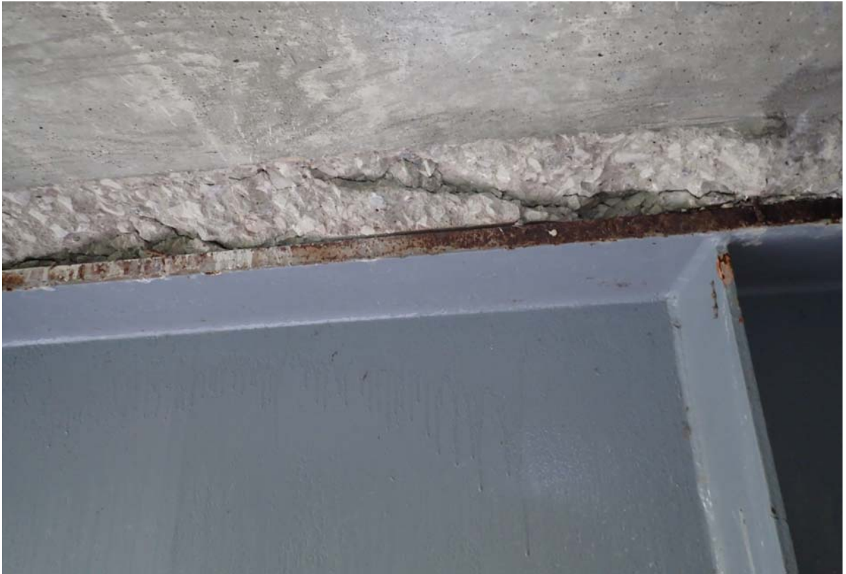
View of moderate cracking and spalling of the fillet above the upstream girder in span 1.
