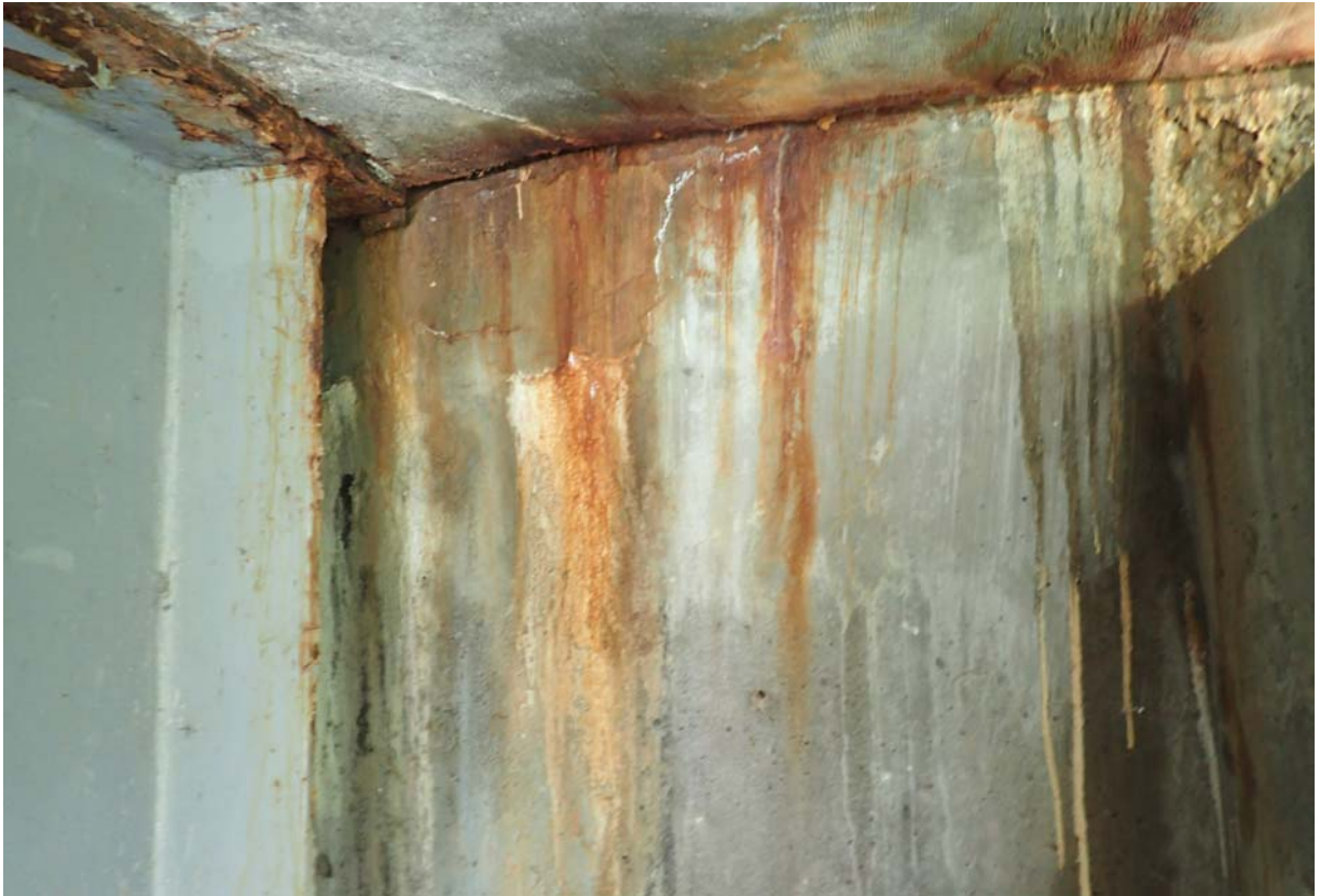
View of minor cracking with efflorescence along the downstream backwall of abutment 1.
