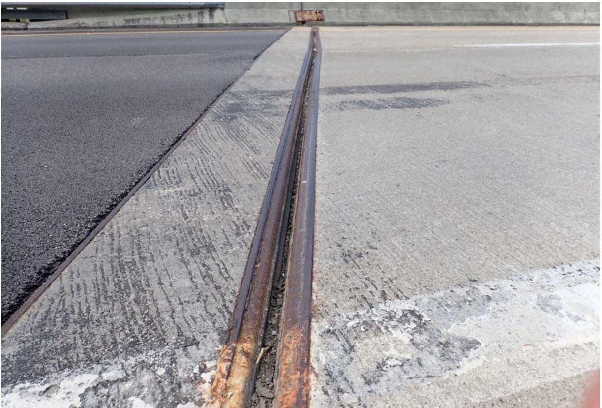
View of the transverse joint at abutment 4. It is mostly full of dirt and debris.
