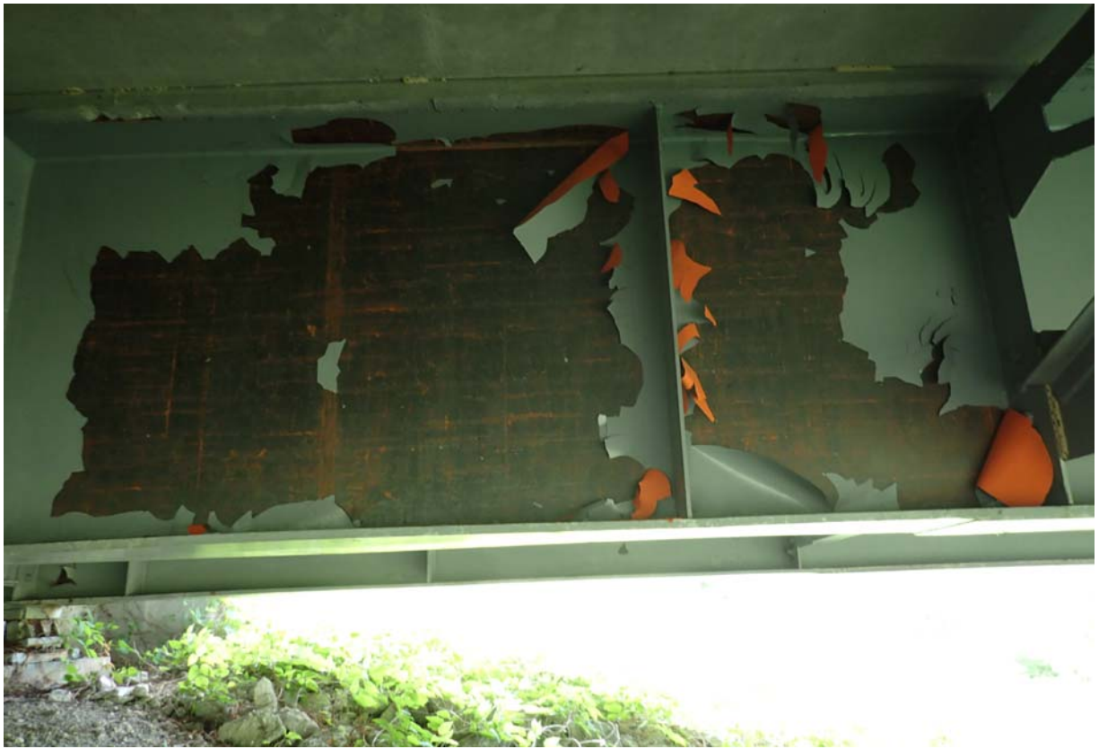
Large areas of paint failure on the downstream face of girder 2 in span 3.
