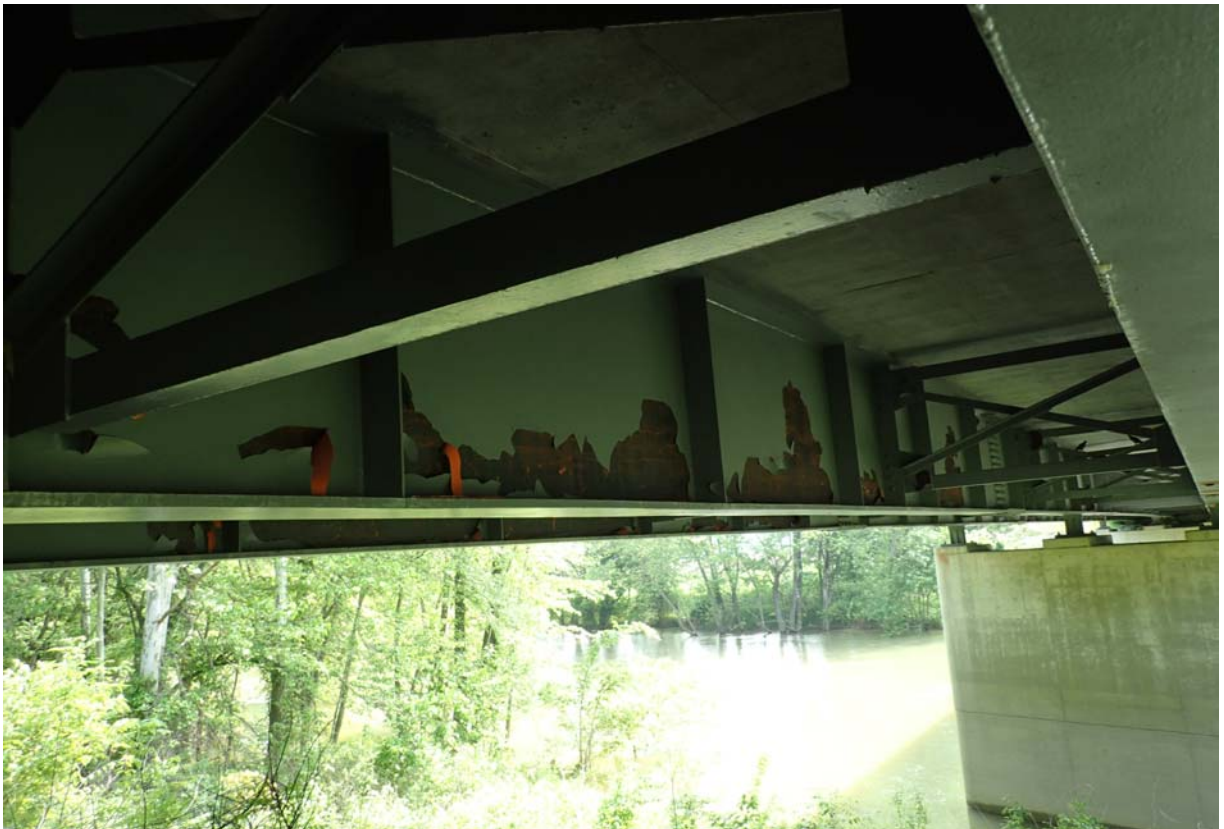
View of several large areas of paint failure on the upstream face of girder 3 from upstream in span 1.
