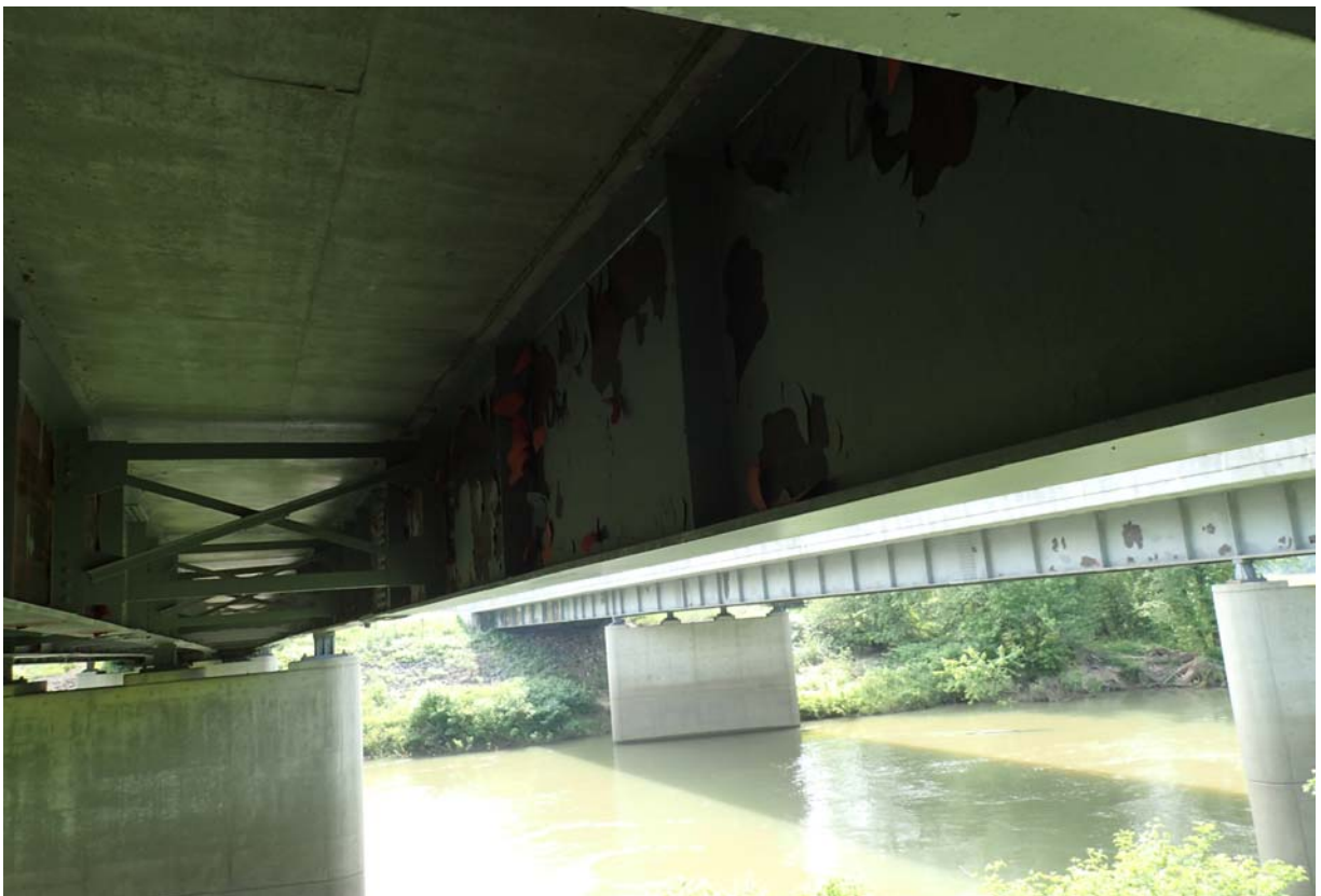
View of several large areas of paint failure on the downstream face of the upstream girder in span 1.
