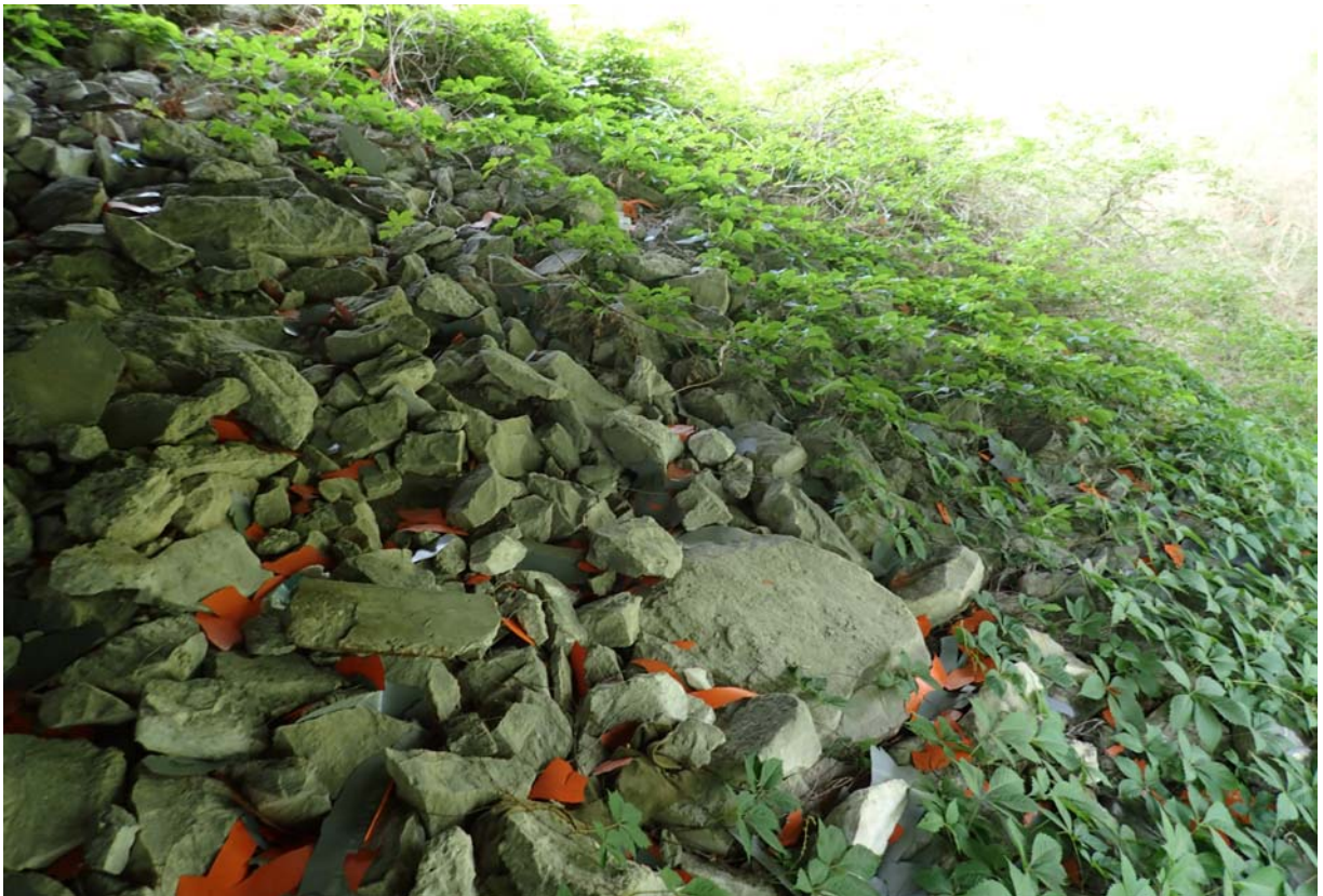
View of paint lying on the ground near abutment 4.
