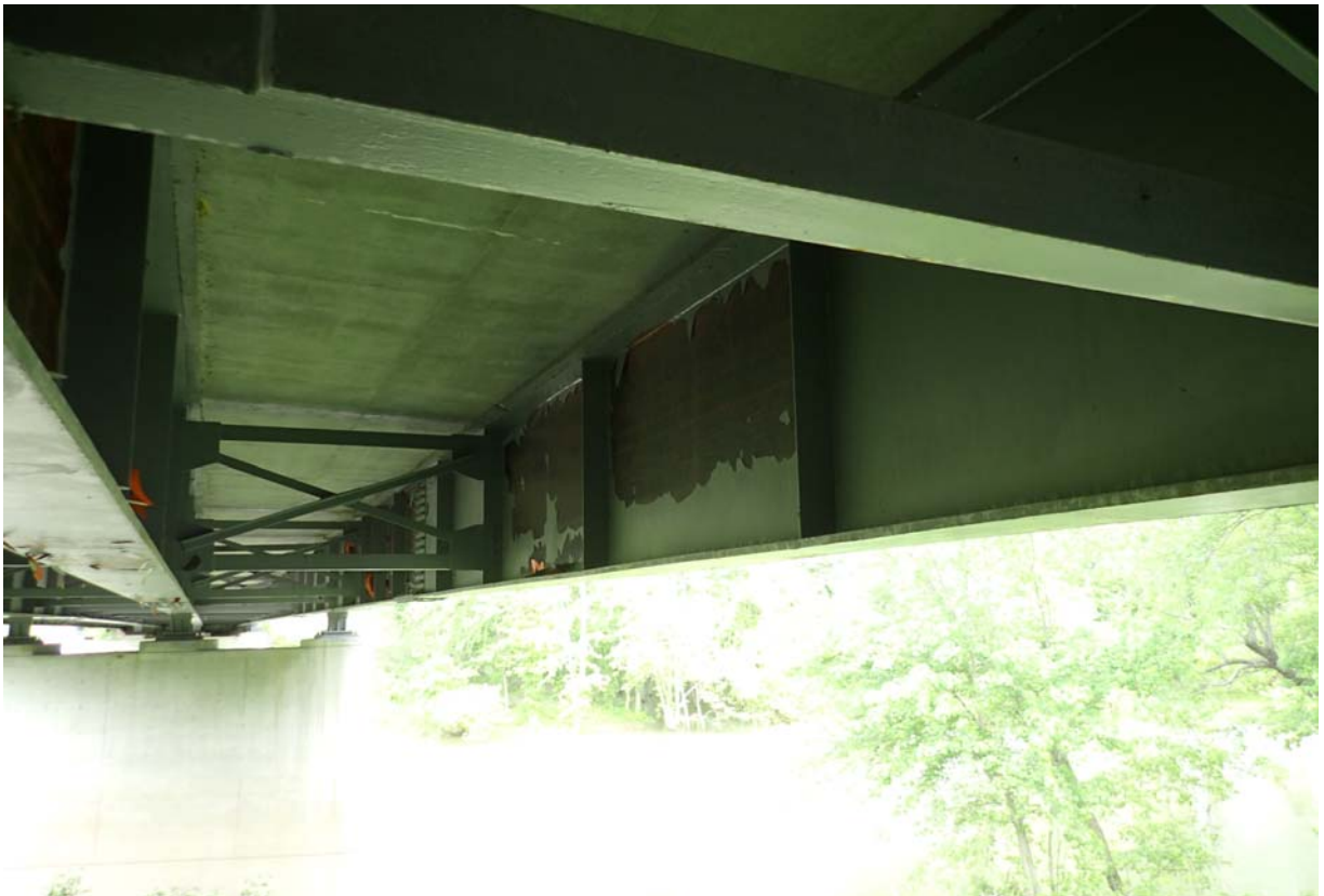
Large areas of paint failure on the upstream face of the downstream girder in span 3.
