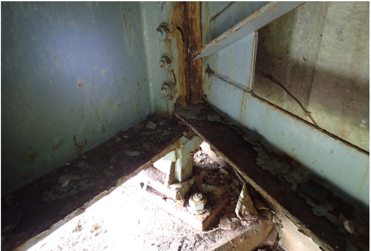
View of flaking paint and moderate corrosion at the end of the upstream girder at abutment 1.
